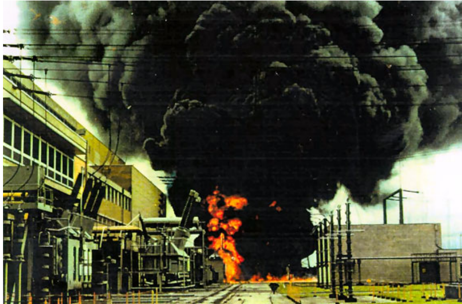
Figure 8-6: Transformer fault due to a defective bushing
